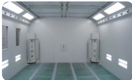
Air supply units for painting and varnishing chambers.
